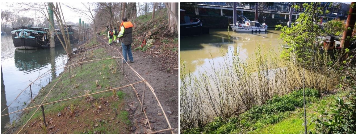
Planting carried out by the association Espaces along a 150-metre stretch of the Seine at l'île de Puteaux. ©Association Espaces
