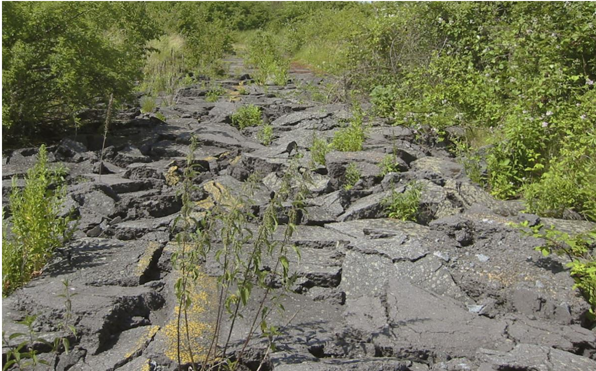
Breaking up concrete prior to natural regeneration at the former Bonames Airport (Frankfurt, Germany) © GTL, Michael Triebswetter
